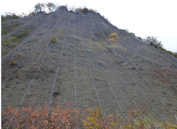
写真-1.1 覆式落石防護網
