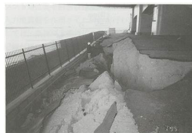
写真 1.2.2.10 新夙川橋の護岸付近の地表面のひび割れ Photo. 1.2.2.10 Crack of ground surface around shore protection of Shin-Shukugawa Bridge
