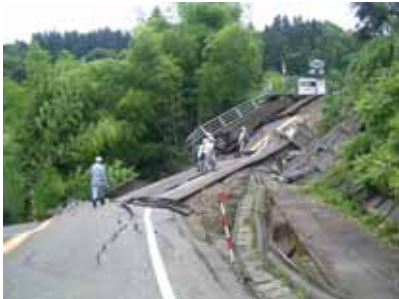
PWRI's researchers conducting investigation at Chuetsu Offshore earthquake disaster site.
