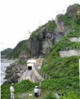
Technological support applying emergency measurement techniques at the collapse site in Noto Peninsula earthquake.
