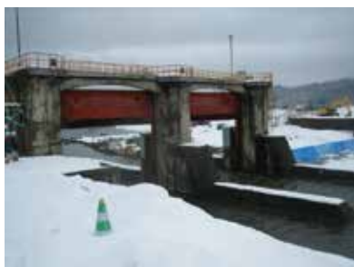
Example of deterioration of irrigation facilities: pier of the headworks with wear and frost damage, and gate with wear and corrosion
