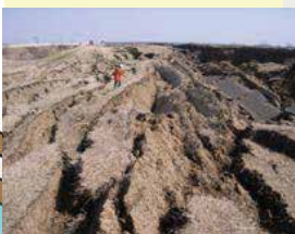
Emergency responses to large-scale damage of river embankments and floods
