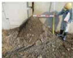
Example of outflow of reinforced-back-surface soil (a simple maintenance method is required)
