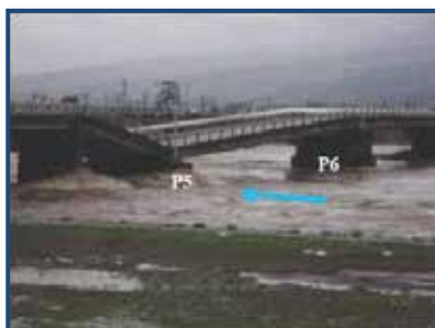
Local scour around bridge piers
