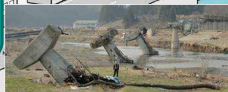
Loss of bridges and damage to substructures caused by tsunami
