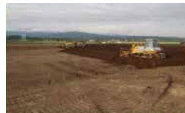
Construction of large-sized paddy field: Decision on selection of machinery and construction timeframe based on the soil diagnosis is required.
