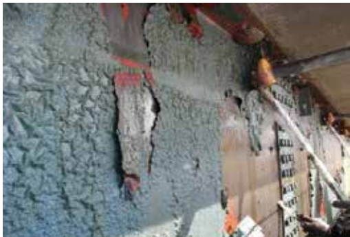
Coating film being peeled off
