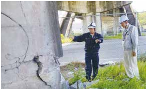
Kumamoto Earthquake: Inspection of damages at the crossover in the City Road Chuo Line (17 Apr.)
