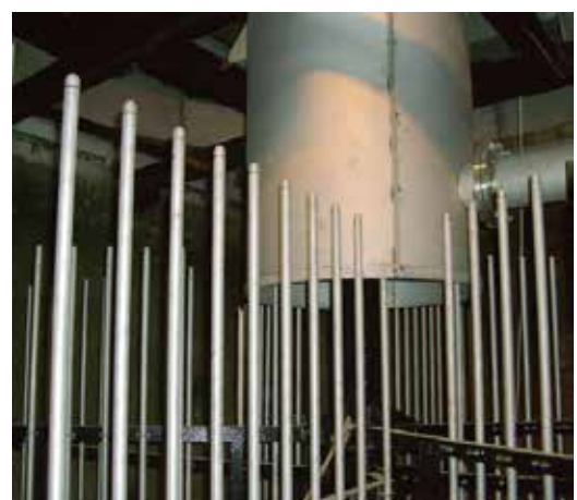
WPFs installed at the Engaru Wastewater Treatment Plant
