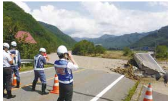
Typhoon No.10 etc.: Field survey of the collapsed bridge in Hidaka Town (1 Sep.)
