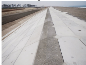
Completed part of the seawall near the Sendai Airport (left: land side)
