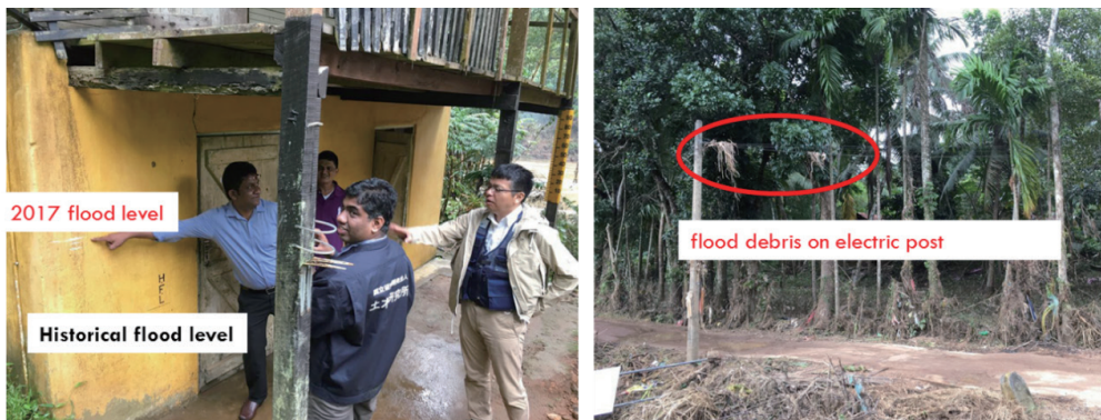
Fig. 4 Field survey of flood levels in the affected areas with guidance of Irrigation department (Chief Eng. SPC Sugeeshwara).
