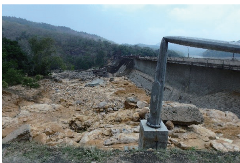
Poringalkuthu Dam and its downstream erosion of the left bank Poringalkuthu ダムとその直下左岸側の侵食被害
