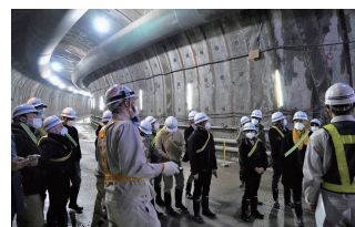
Inside the Kusaka River New Floodway Construction 日下川新規放水路の工事現場にて
