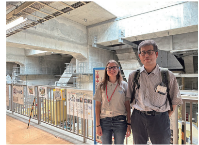
Visit to Metropolitan Area Outer Underground Discharge Channel (Saitama pref.) with Ushiyama-sensei
