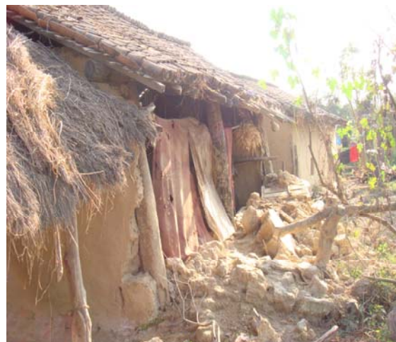
Fig. 2.6 Scene of damaged thatched house in Mahadevnager
