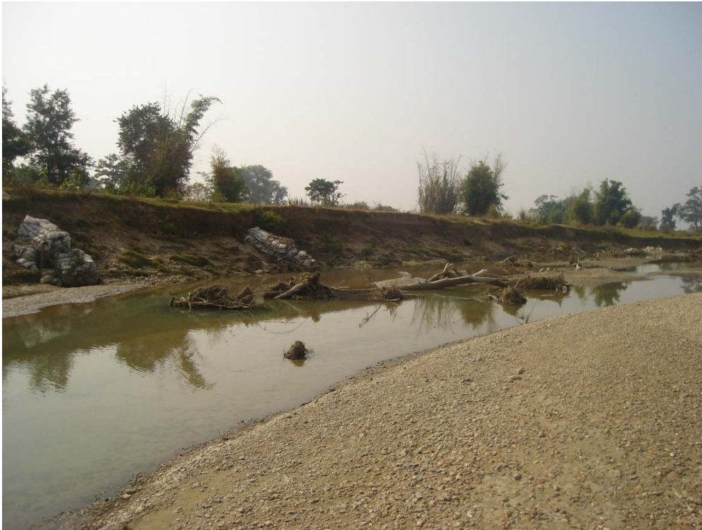
Photo 6 Failure of Spurs
