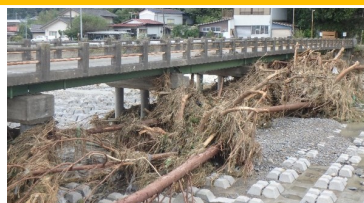
A scene from an investigation on damage caused by Typhoon No. 19 in 2019 (Tochigi Prefecture, Japan)
