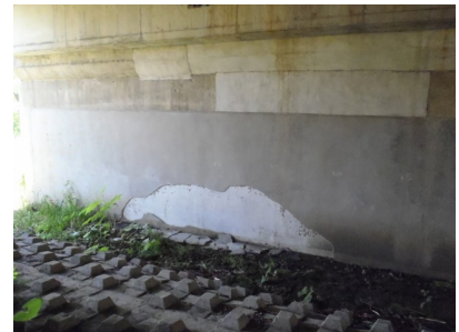
(c) 浮き箇所の剥落
