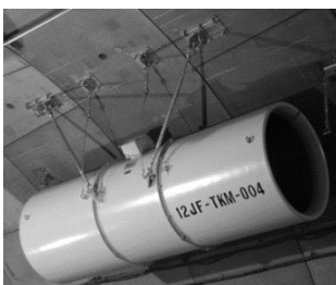
Photo-1: Jet fan in road tunnel
