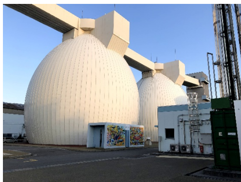
Photograph1: Example of the digestion tank (Higashinada WWTP in Kobe City)
