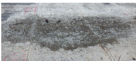
Photograph 1: Disintegrated concrete beneath asphalt surfacing in RC bridge deck slabs
