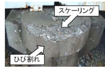
Typical case of frost damage
