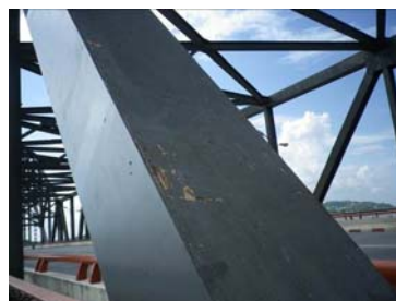
Deterioration of paint on Ayeyarwardy bridge
