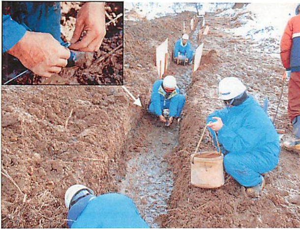
写真-5 地表面変位計測用光ファイバ敷設状況 Photo.5 Setting of Optical fiber sensor for measurement of the ground surface
